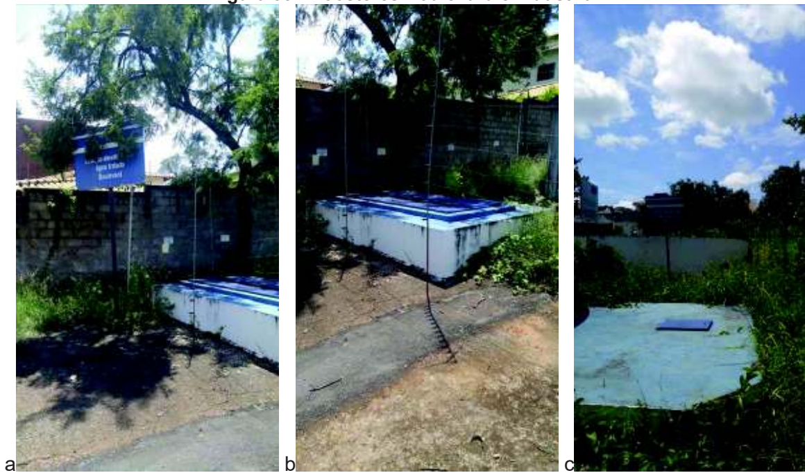
Figura 55 - Boosteres Boulevard e Industrial
